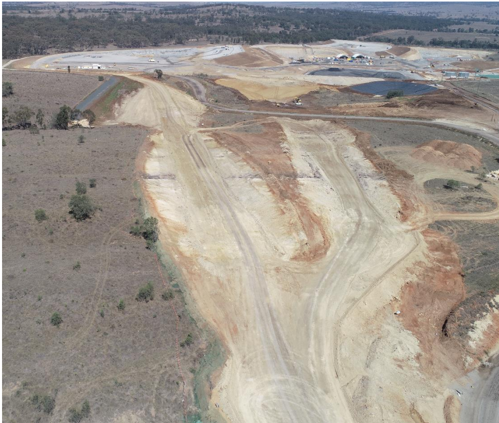
Conveyor Trace – September 23
