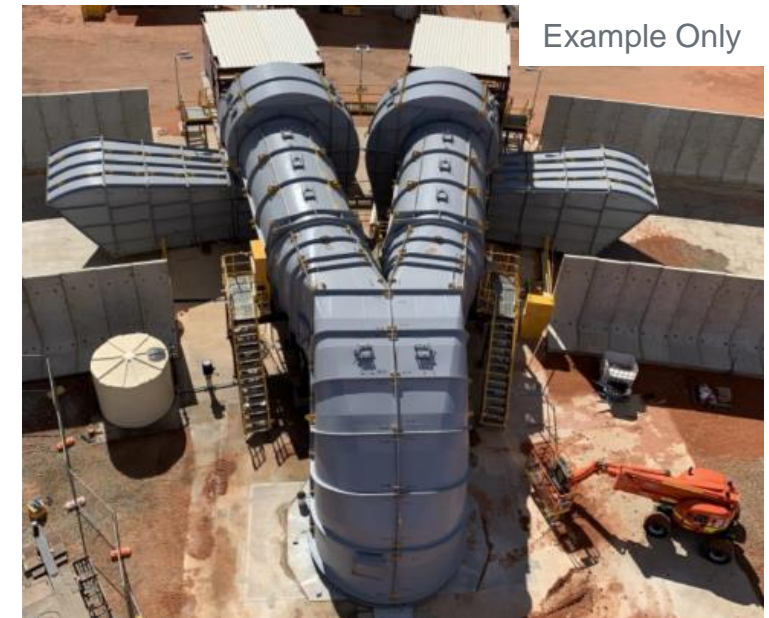
Low-profile ventilation ducts so that the maximum height is only 9.5 m above ground
