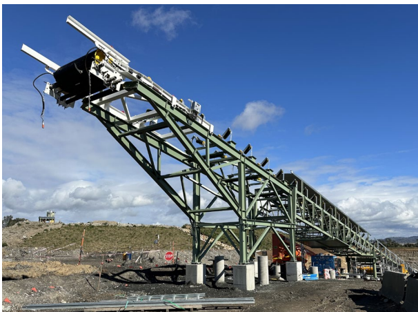
Longwall drift conveyor
