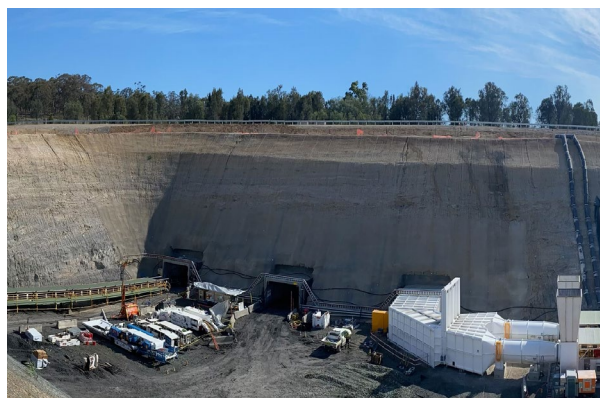
B&P portal showing permanent ventilation system
