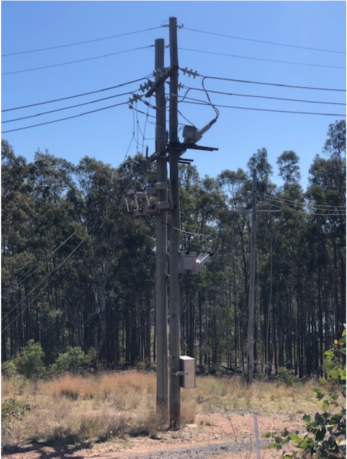
Figure 1-4 Existing 33kV transmission line metering point adjacent to Maxwell Infrastructure substation
