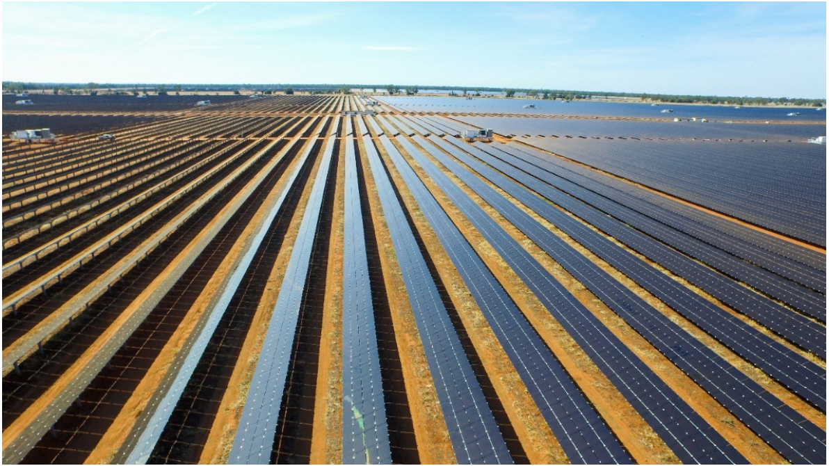
Figure 4-1 Typical fixed array solar plant - Nyngan NSW (Nyngan Solar Plant is owned by the Powering Australian Renewables Fund (PARF). Image courtesy of PARF)
