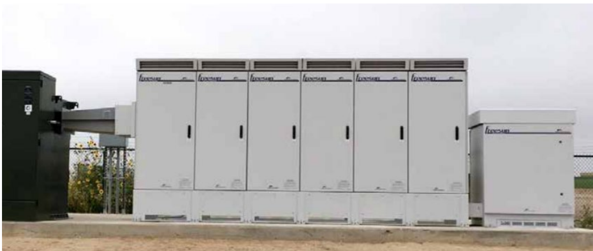
Figure 4-6 Typical PCS (courtesy: Power Electronics)
