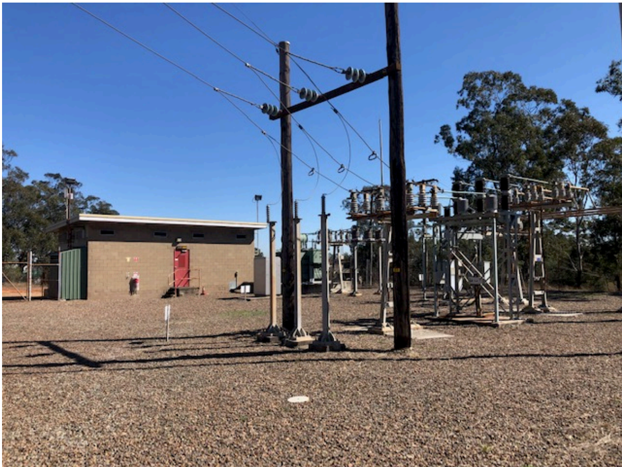
Figure 1-3 Existing Maxwell Infrastructure substation and associated infrastructure
