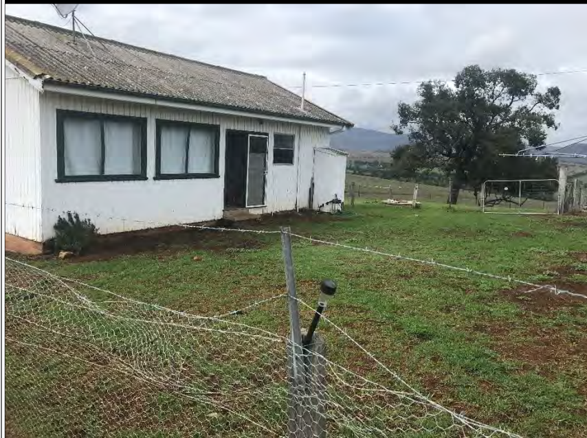
PHOTOGRAPH Z: RESIDENTIAL BUILDING WITH POTENTIAL ACM ROOFING
