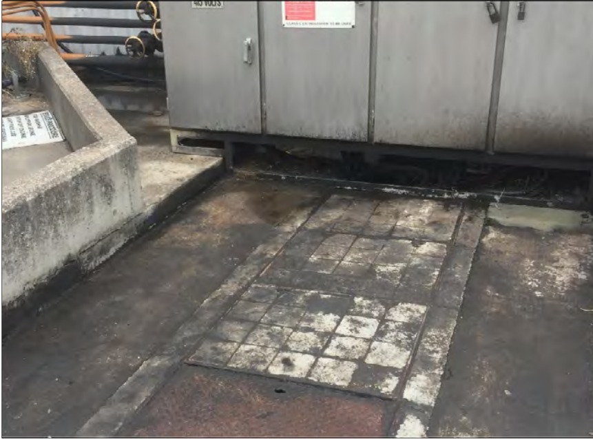
PHOTOGRAPH AK: AFTER CLEAN-UP OF FUEL SPILL ADJACENT TO ASTS (PROVIDED BY MALABAR COAL)
