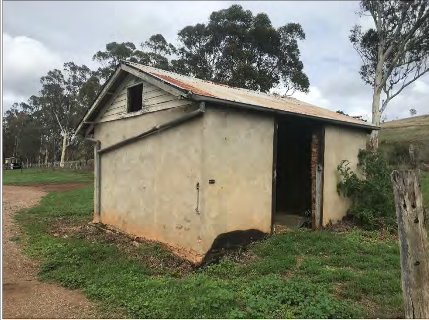
PHOTOGRAPH V: CONCRETE / TIMBER STABLE, BLACK STAINING
