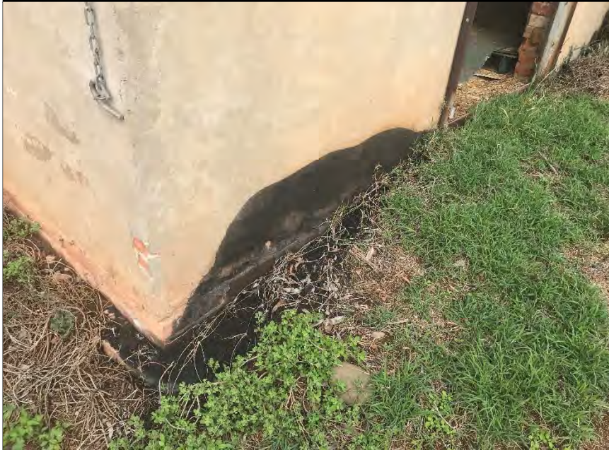
PHOTOGRAPH W: STABLE, BLACK STAINING
