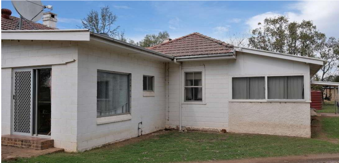
Figure 31 – View of the south-east corner of Bowfield, showing the hip roof of the second wing constructed in off form concrete with an embossed block pattern and timber sash window dating to the c.1950s. The skillion roofed wing at the left is part of the c.1960s front wing of the homestead.
