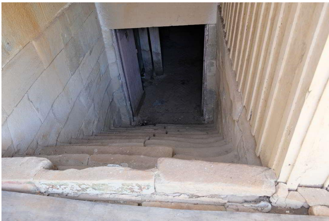
Figure 52 – View of stone stairs leading down to the cellar at Plashett Homestead.
