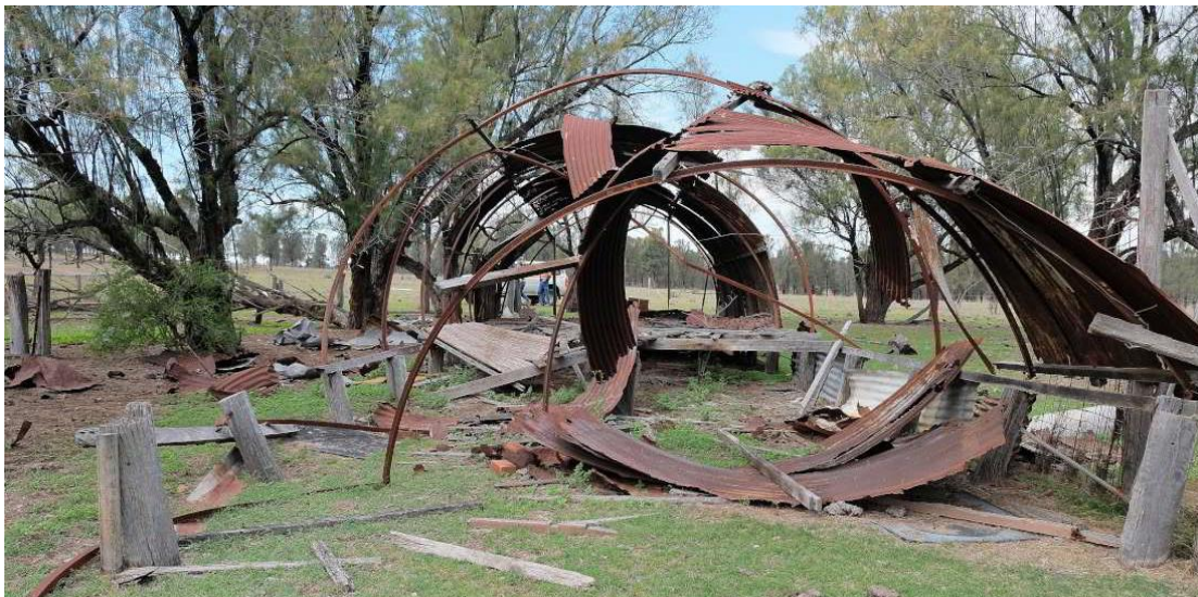
Figure 36 – View of the collapsed rear (southern end) of the Nissen Hut with only the perimeter posts remaining in their original location. The flooring is completely missing with only a small area of collapsed roofing existing.
