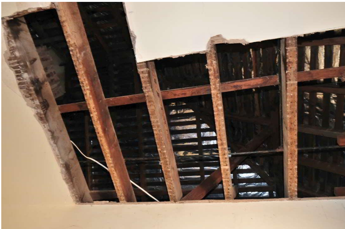
Figure 55 – View up through ceiling space in Plashett Homestead showing closely spaced roof battens indicative of slate roof cladding at time of construction.
