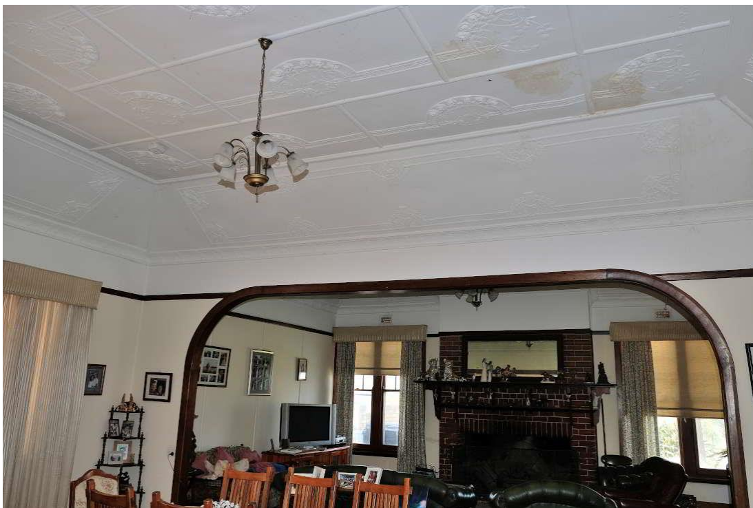
Figure 23 – The generous dining and living room areas are divided by a wall with a wide opening, featuring arched corners. This detail is repeated throughout the dwelling at several doorways.
