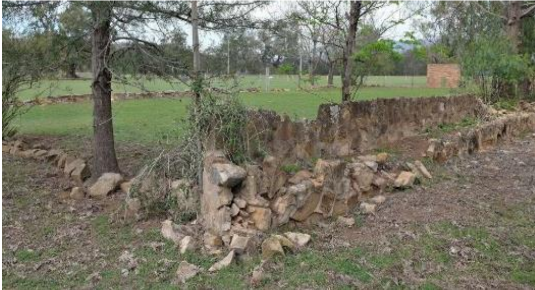
Figure 26 – View of the collapsed rock-edged garden beds around the former tennis court.
