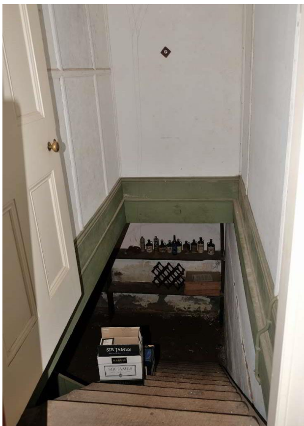
Figure 21 – View of stairwell in the eastern wall of former ballroom providing access to cellar.
