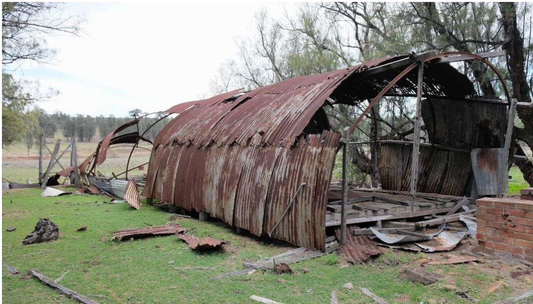
Figure 34 – The Nissen Hut at M04. Some debris of the structure is scattered around the site.
