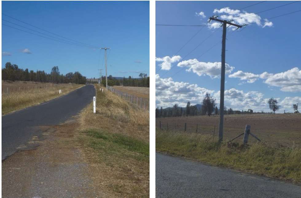
Fig. 6.14 11 kV voltage powerline along Edderton Road
