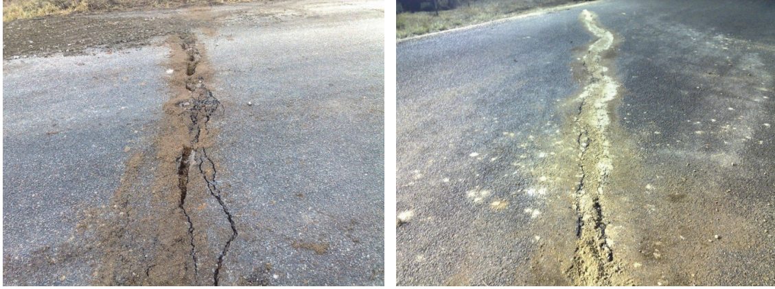
Fig. 6.13 Impacts observed along Charlton Road at the Beltana No. 1 Underground Mine
