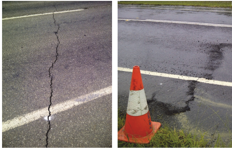
Fig. 6.11 Impacts observed along Broke Road at the Blakefield South Mine
