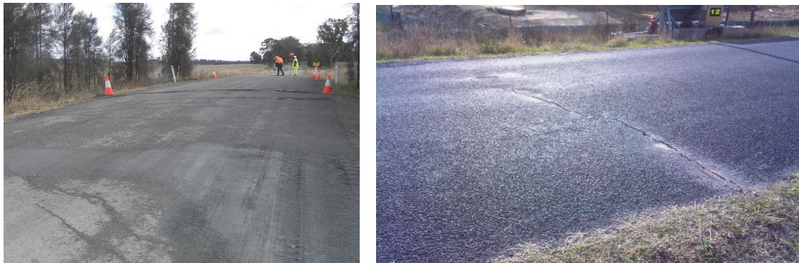
Fig. 6.12 Impacts observed along Charlton Road at the Blakefield South Mine
