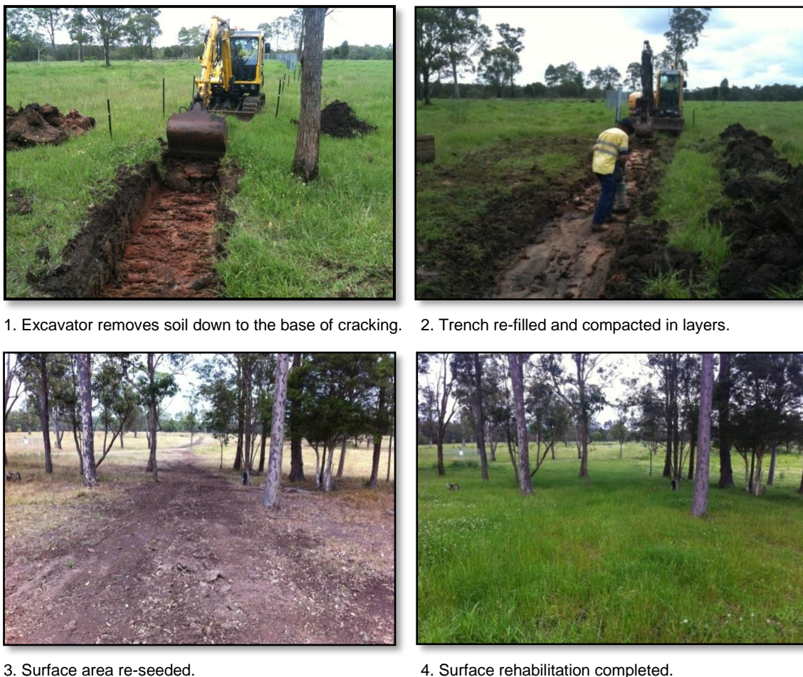
Fig. 4.7 Example of surface crack remediation in the Newcastle Coalfield (Courtesy of Donaldson Coal)
