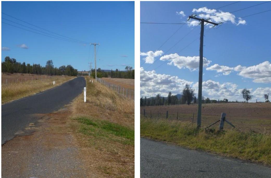
Fig. 6.14 11 kV voltage powerline along Edderton Road
