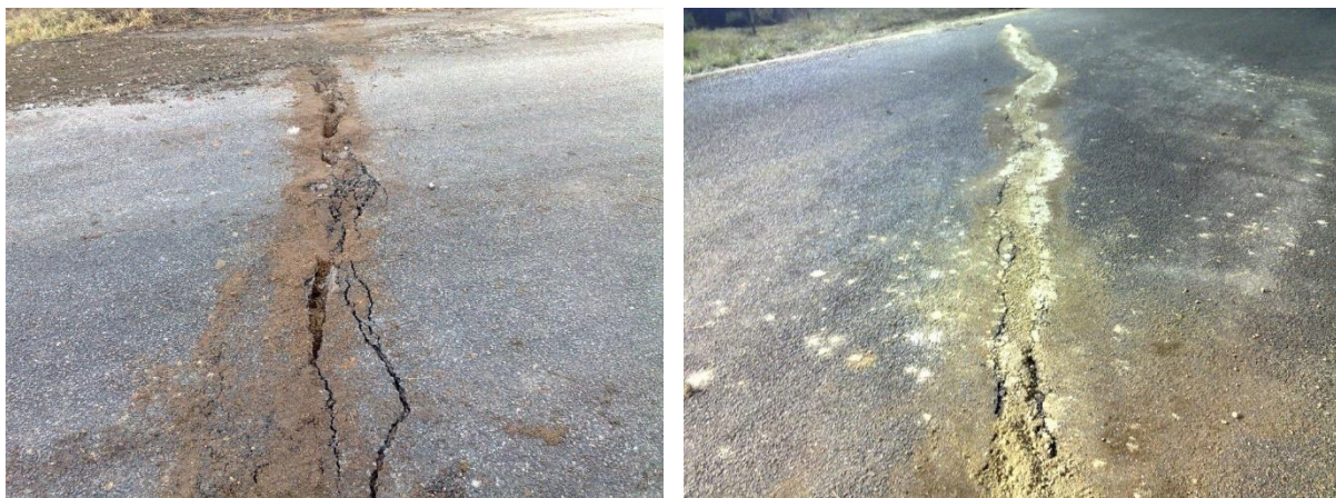
Fig. 6.12 Impacts observed along Charlton Road at the Beltana No. 1 Underground Mine
