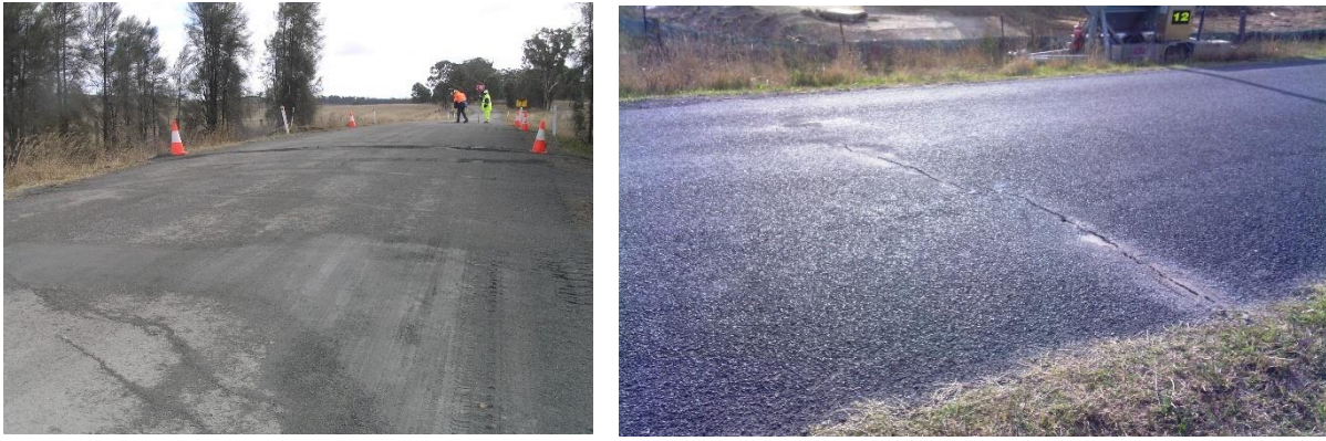
Fig. 6.11 Impacts observed along Charlton Road at the Blakefield South Mine
