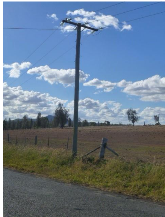
Plate 2: 11 kV voltage powerline along Edderton Road
